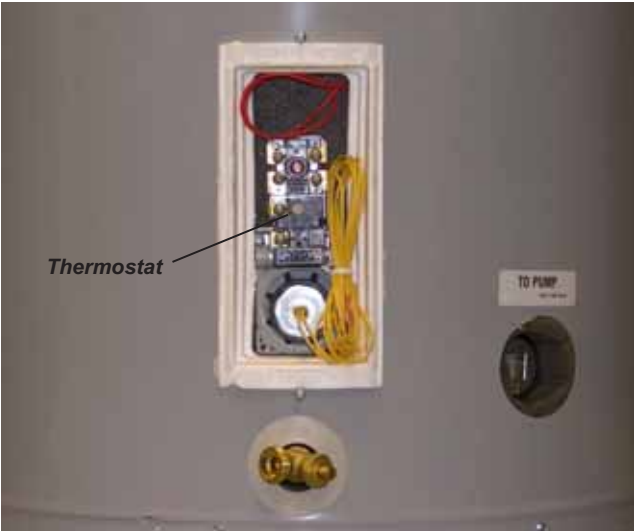
Geothermal storage tank thermostat
